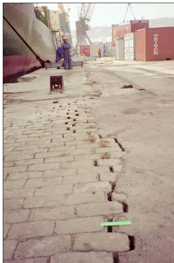
Figure 51 Tension cracks longitudinal to the quay wall indicating lateral wall movement at the Port of Algiers.
