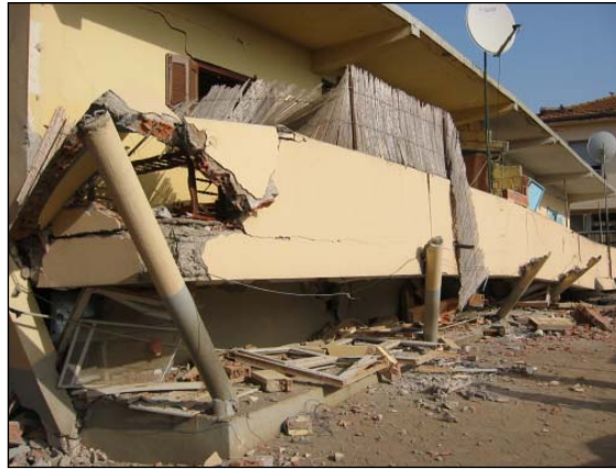
Figure 7 Elementary school in Corso. Insufficient lateral resisting system.
