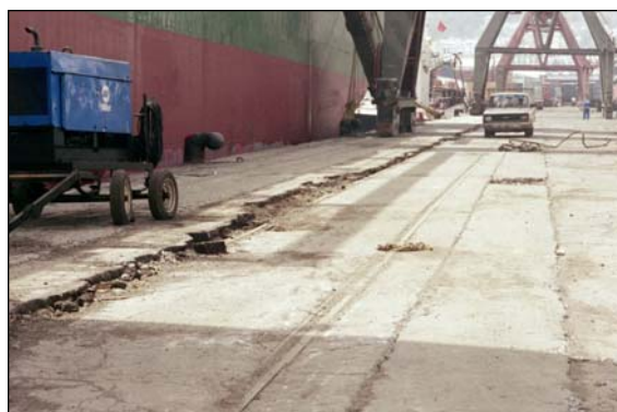
Figure 50 Differential settlement between quay wall and backland, Port of Algiers (vertical offset away from the water).
