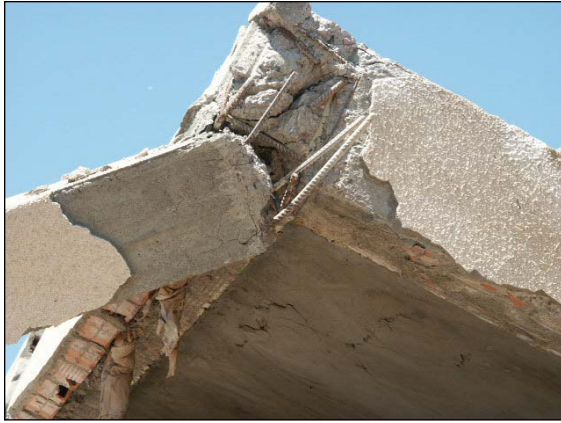
Figure 31 Shearing of corner column due to lack of transverse confinement and poor seismic detailing.
