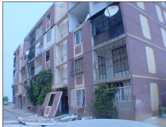
Figure 34 Failure of precast façade elements in cast-in-place concrete tunnel buildings.
