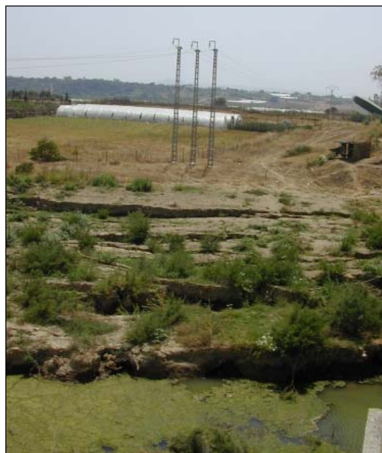
Figure 22 Liquefaction-induced lateral spreading of the banks of Isser River.
