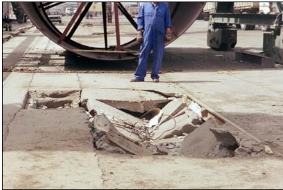
Figure 52 Loss of ground support under concrete pavement at the Port of Algiers.
