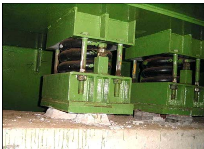
Figure 42 Good performance of vibration isolators.
