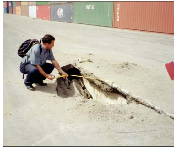
Figure 53 Cavity caused by loss of soil support due to liquefaction at the Port of Algiers.
