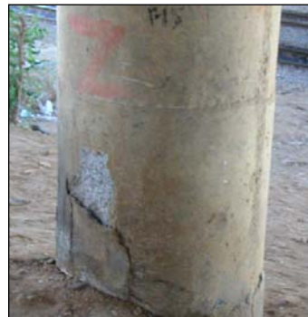
Figures 48a and b Typical minor, localized damage to bridge structures.
