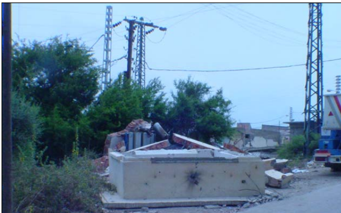
Figure 17 Concrete cap thrown from its original location.
