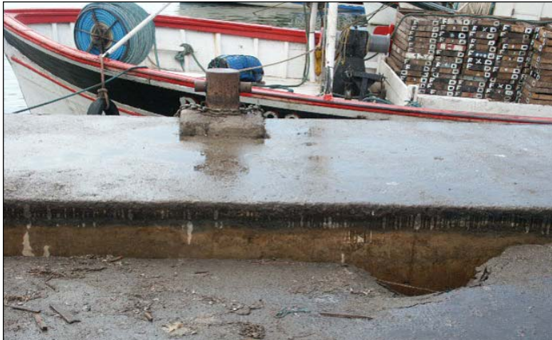
Figure 54 Settlement (>0.3 m) behind pier in the harbor of Zemmouri El-Bahri (close to the epicenter).
