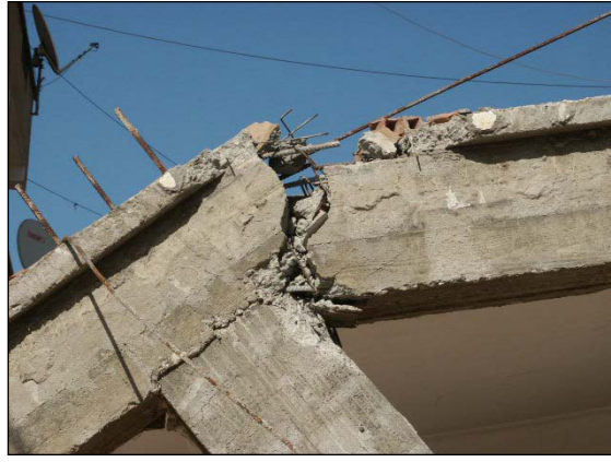
Figure 32 Failure of beam at beam-column due to lack of development of reinforcement and insufficient ductility.
