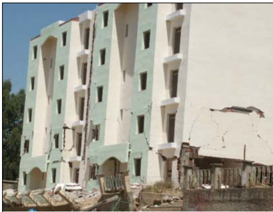
Figure 33 Failure of masonry infill walls.
