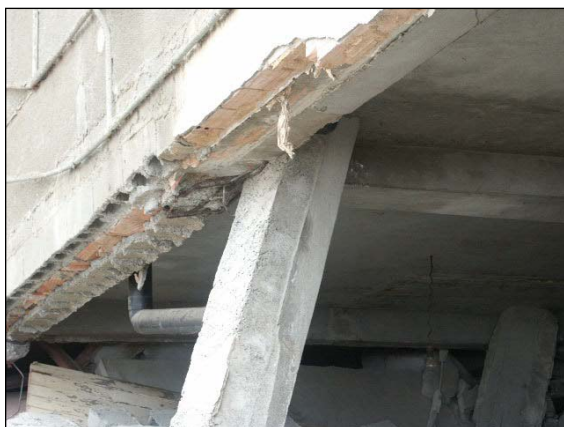
Figure 27 Shearing of column at top of first floor of a residential building.
