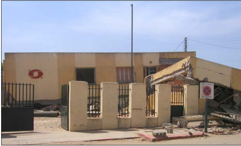
Figure 44 Collapsed telecommunications center in Zemmouri.
