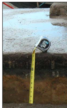
Figures 55a and b Additional views of settlement behind pier in the Harbor of Zemmouri- El-Bahri
