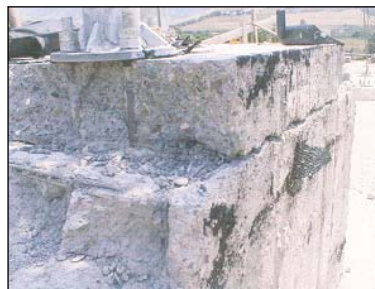
Figures 45a and b Typical anchorage failure of antenna.
