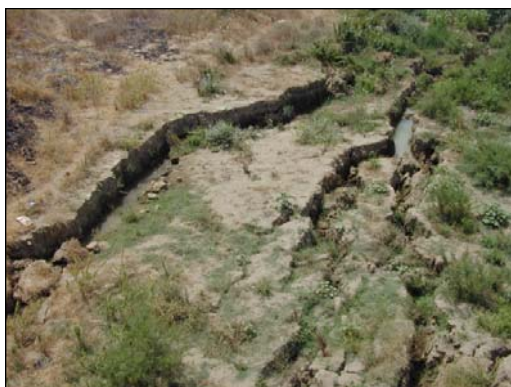
Figure 23 Close-up view of tension cracks caused by lateral spreading of the river bank.
