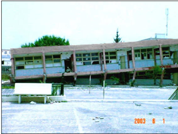
Figure 6 First floor collapse of school building in Boumerdes.
