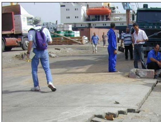
Figure 49 Differential settlement between the quay walls and backland, Port of Algiers (vertical offset toward the water).
