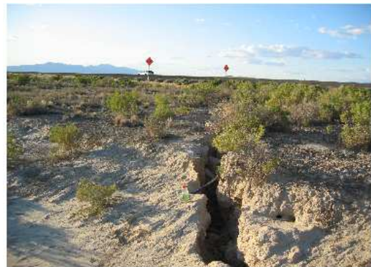
Figure 15: Damage caused by groundwater extraction. The examples are a house in the Las Vegas area (upper and middle picture) severely damaged by soil subsidence due to groundwater extraction, and a major highway in Northern Nevada damaged by soil cracks and subsidence resulting from lowering the groundwater level for mining (lower picture). Courtesy John Bell.
